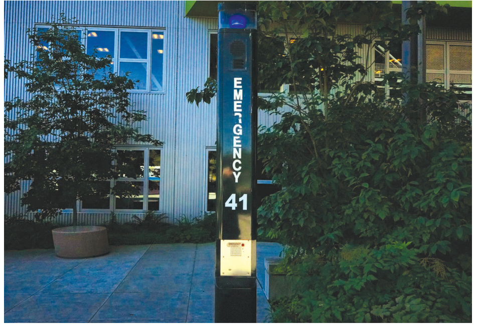
Emergency line 41, Activities and Recreation Center (ARC Building)
